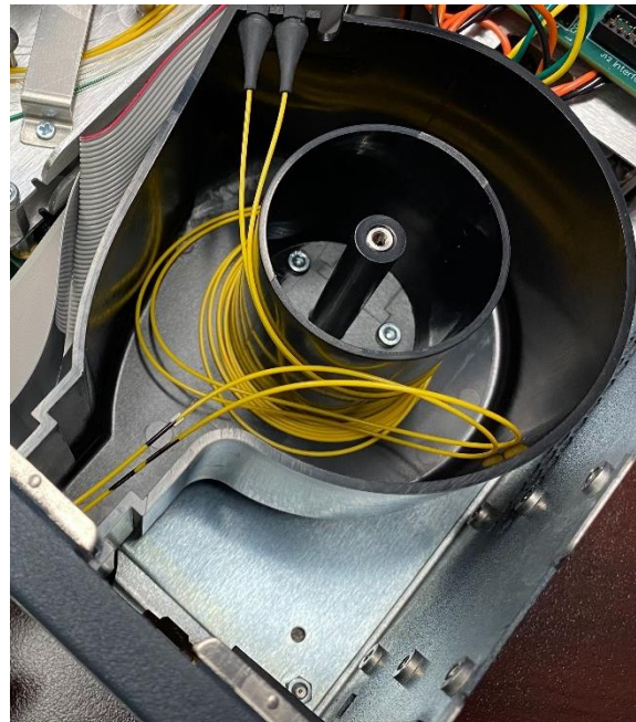
Figure 20: Exposed view of poor output fiber management
